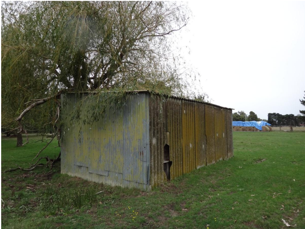
Photograph 144: Former stock shelter potential asbestos cement wall.
