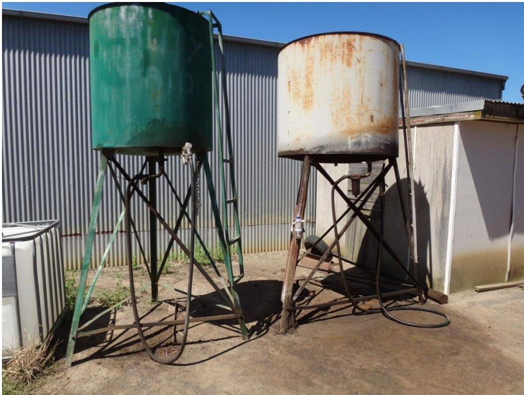
Photograph 81: Diesel ASTs located in the south west portion adjacent to a storage shed and vegetable washing shed.
