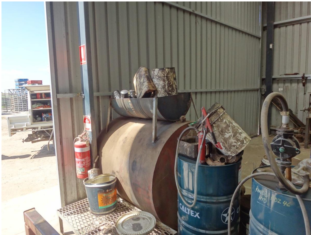
Photograph 127: Waste oil AST located in the vehicle maintenance shed.
