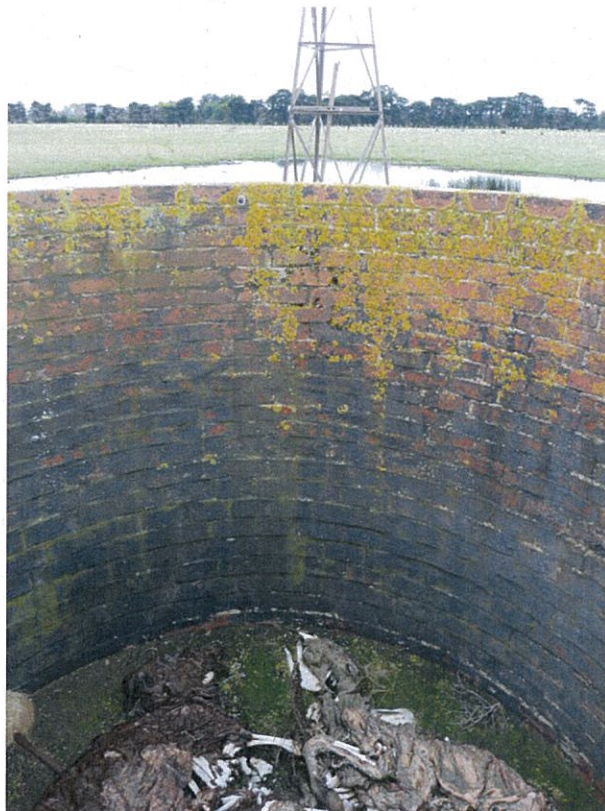
Photograph 10: View of carcasses found inside a disused water tank adjacent to the dam in the east portion of the site.
