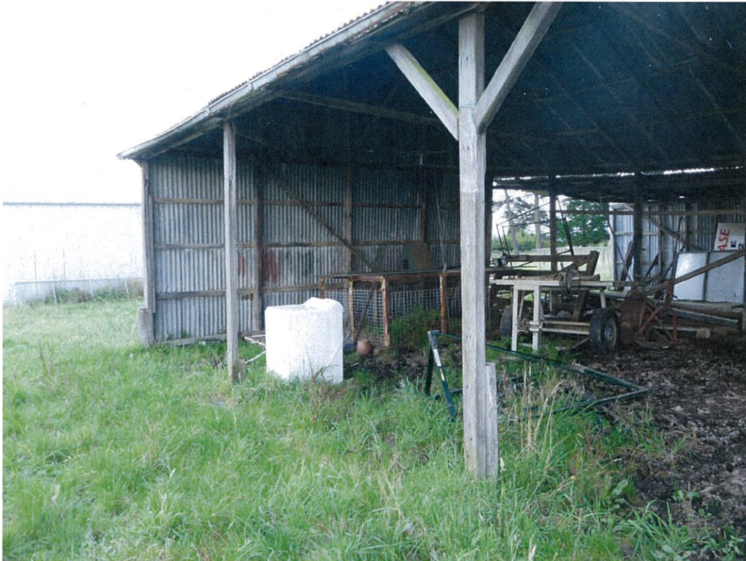
Photograph 15: Farm machinery shed. Asbestos roofing was found covering the rear of the shed.
