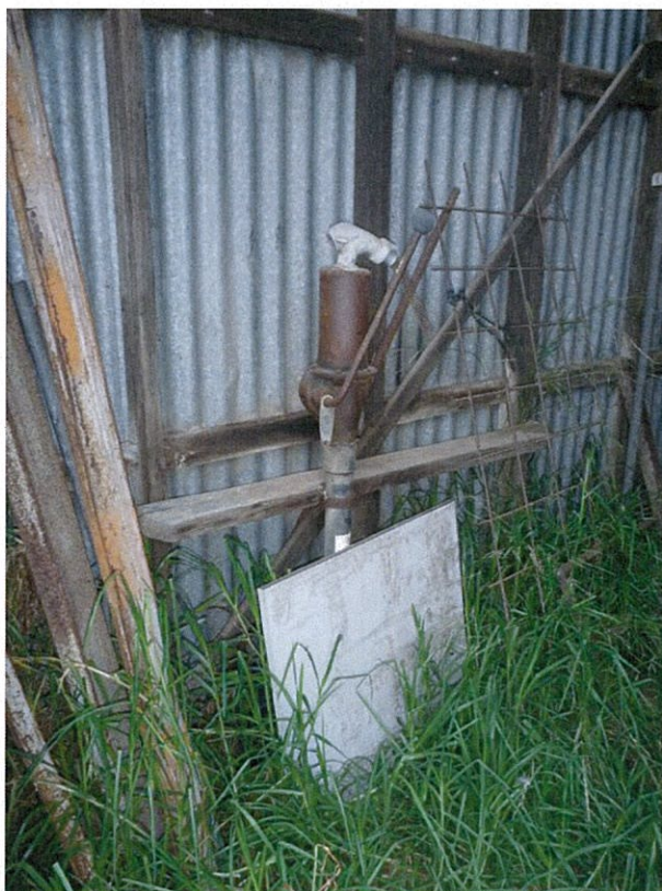
Photograph 11: Underground Storage Tank (UST) hand pump and breather located in farm storage shed. This UST was understood to be no longer in use.
