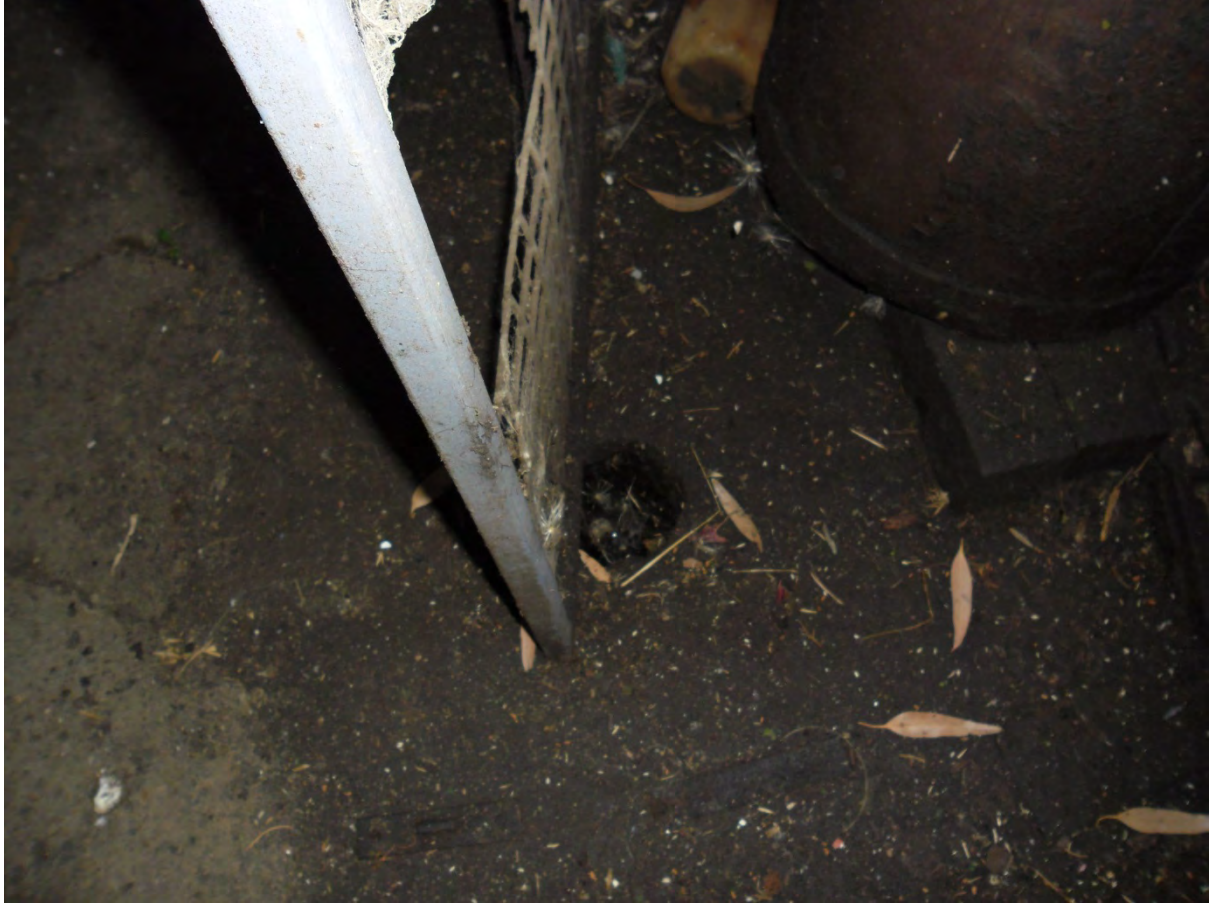
Photograph 15 - Bore hole in dairy building surrounded by oil-stained dirt
