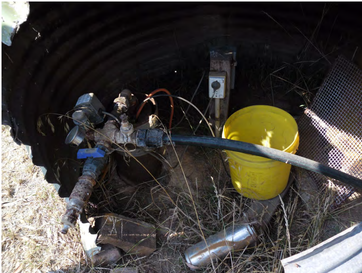
Photograph 13 – Bore with electric pump located at 2040 Mickleham Rd
