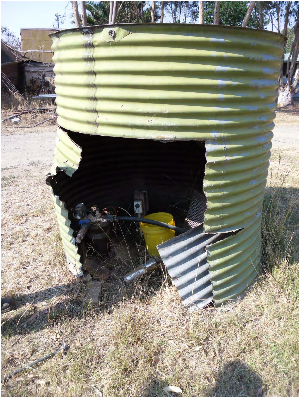
Photograph 12 – Bore with electric pump located at 2040 Mickleham Rd (facing SW)
