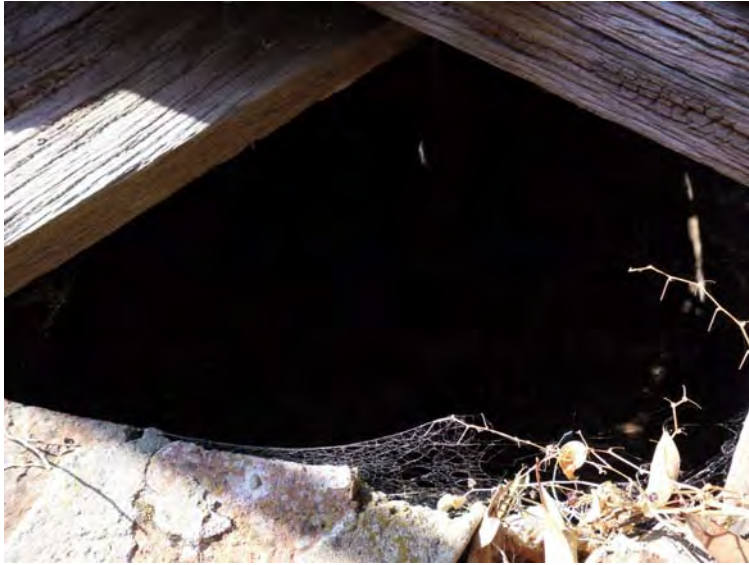
Photograph 09 – View down open well adjacent to septic tank, 2040 Mickleham Rd
