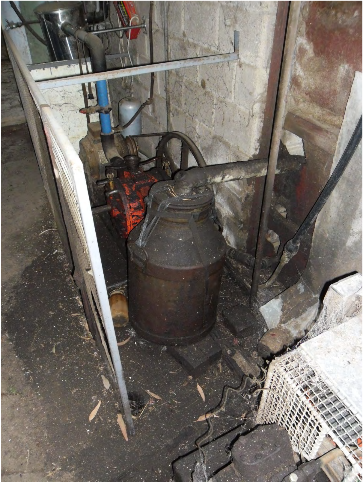
Photograph 14 – Bore hole located in dairy building at 2040 Mickleham Rd
