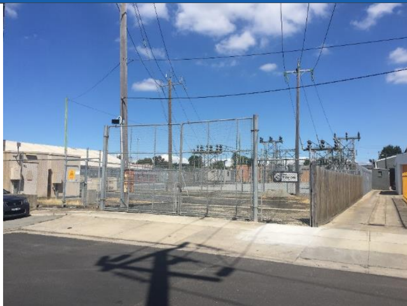
Plate 3 – Looking east towards Power substation/ transformer yard
