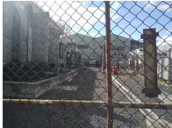
Photo 20. Property 109, Electrical substation
