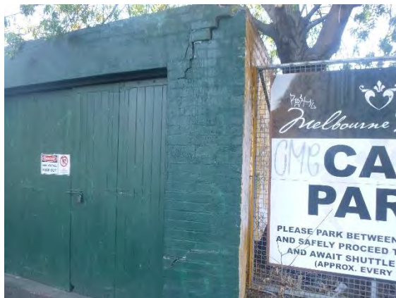
Photo 5. Property 29, electrical substation
