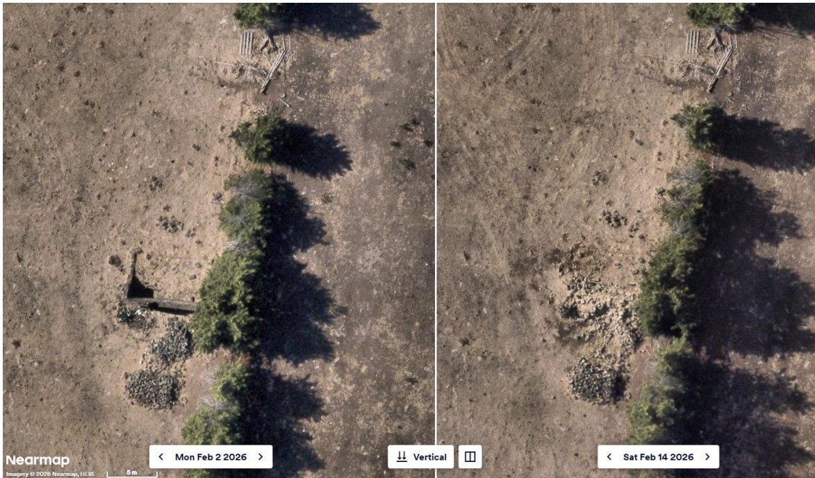
Figure 28 Bleak house ruin showing collapse between 2/2/26 and 14/2/26 (NearMap image)
